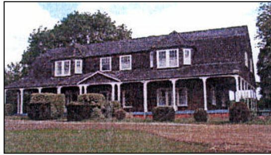
The MacDonal Stewart Pavilion was built in 1897 and is constructed totally of timber with internal and external cladding.
